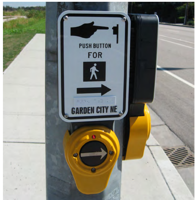
Accessible Pedestrian Crosswalk Signal
