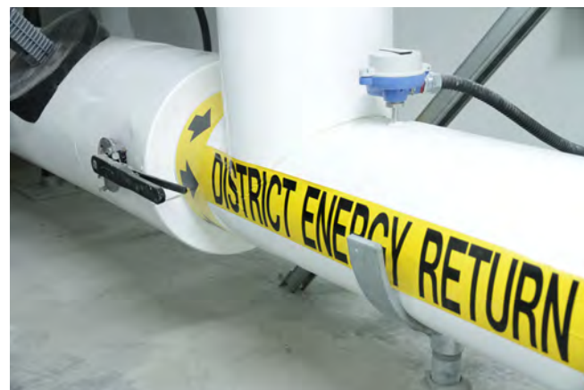
District Energy Utility
