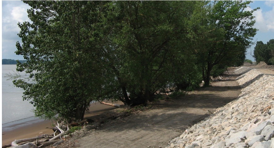
Before and after a dike improvement project which enhanced intertidal habitat and the City's flood protection defences
